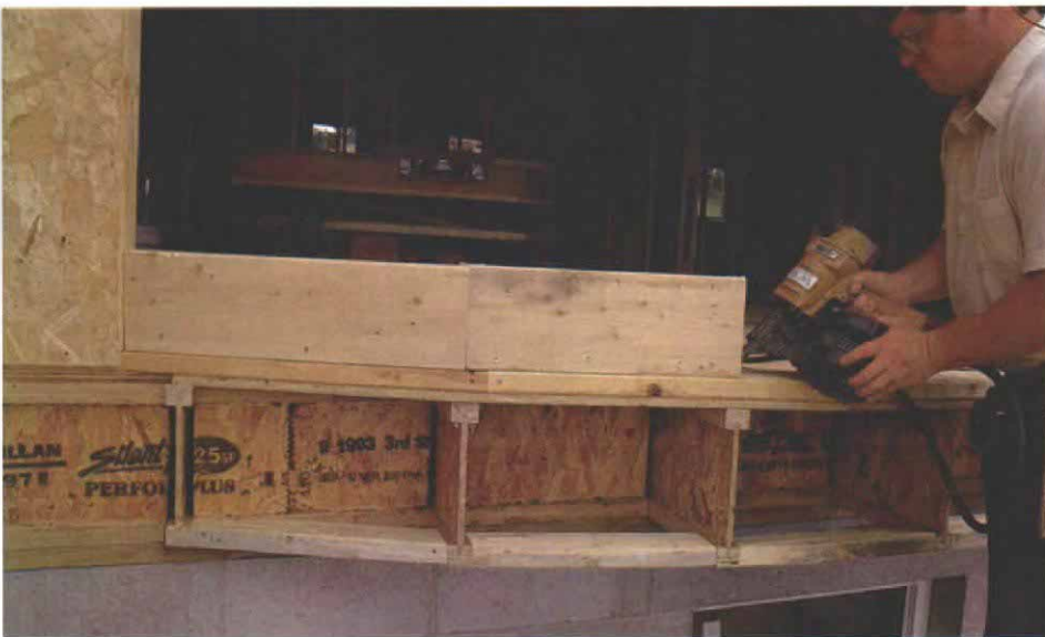
Spanning from joist to joist. The window junctions, which are the weakest points of the unit, don't occur over the floor joists, so doubled 2x8 headers were installed to transfer window loads to the floor joists. These headers are positioned so that they sit within the 2x6 wall plate.
