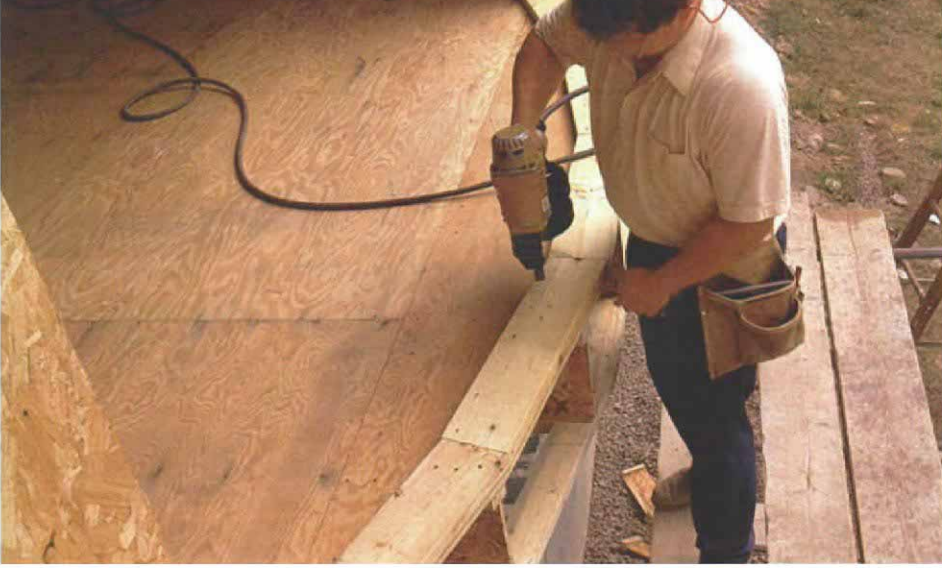
Taking shape. After cutting the joists, 1x4 blocking was nailed along the bottom of the joists to continue the window profile. Then the plywood subfloor was glued and nailed to the joists, and the 2x6 wall plates were measured right from the shape of the subfloor and nailed off.
