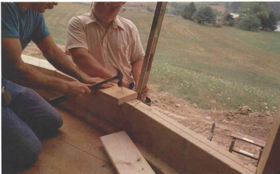
Installing the sill. The walk-out bow window rests on a 2x6 sill; each piece of the sill is identical to the wall plate below it. A level held against the plate indicates when the sill is plumb.
