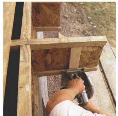
Cutting the cantilever. Floor joists (wood I-beams on 19-in. centers) at the rough opening were left long and then cut to the bow shape. The exact lengths of the joists and angles of the cuts were taken from the drawing.
