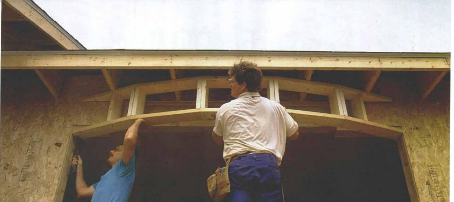
Framing over the window. Because of the house's deep roof overhang, a wall, not a roof, was built above the window. The wall consists of five separate 2x6 frames built to match the window profile. The frames
